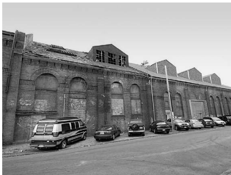
Dilapidated building at 2 52nd Street, Brooklyn, New York
